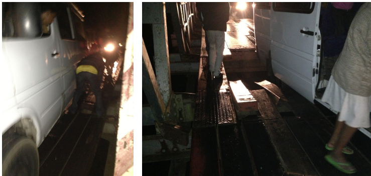
Fig. 6: Taxi brousse being pulled out of a bridge's hole at night (RN 7, Southern Madagascar)
